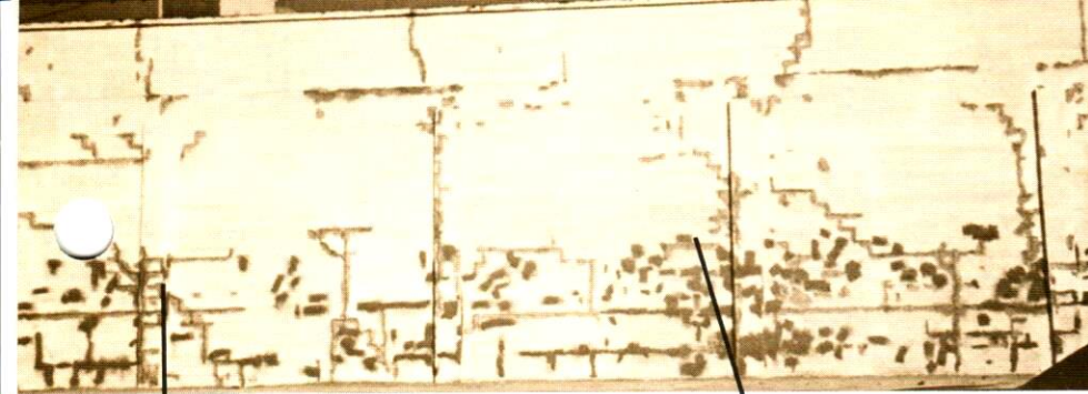
BAD STRUCTURAL DAMAGE CAUSING SEVERE LEAKAGE.
